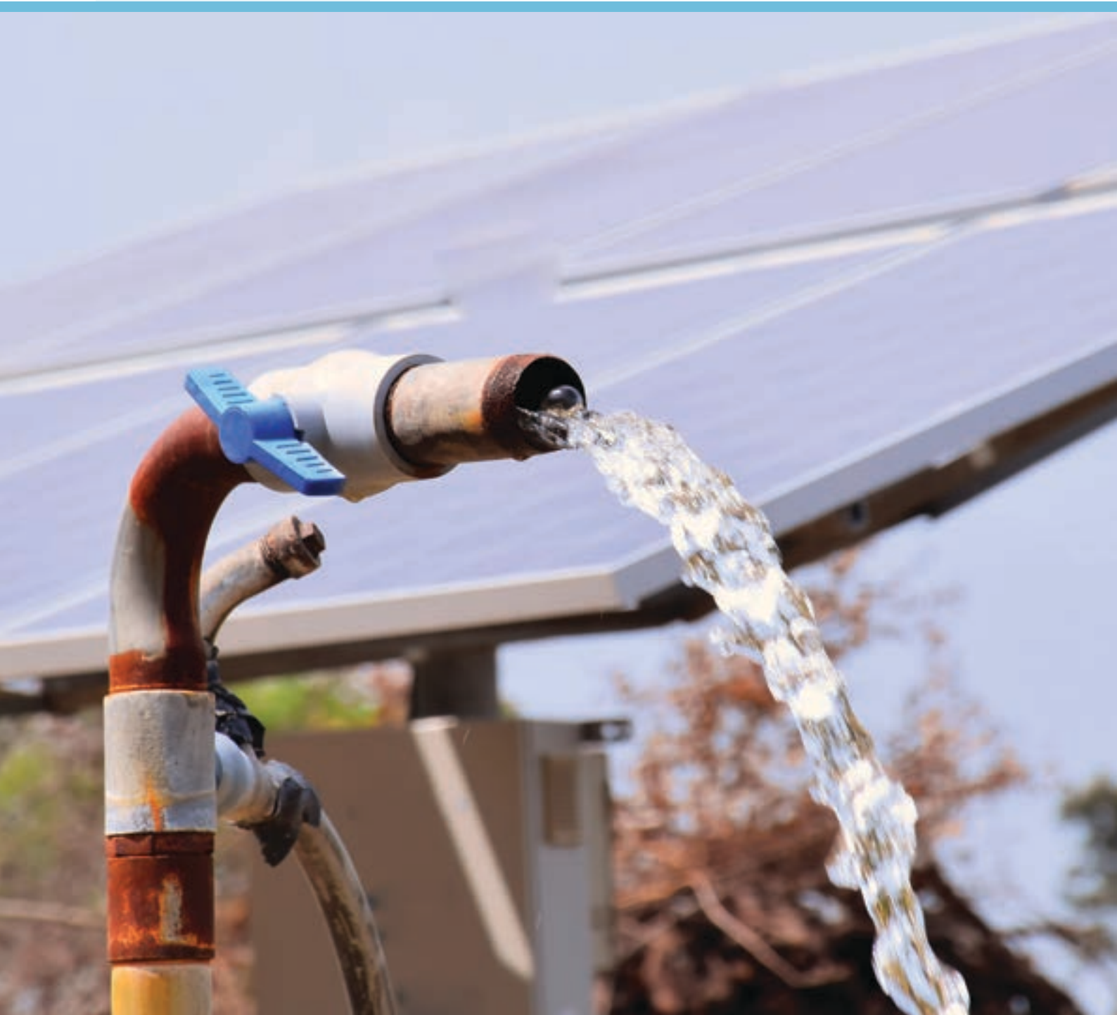
Equipment for a solar-based irrigation project.
